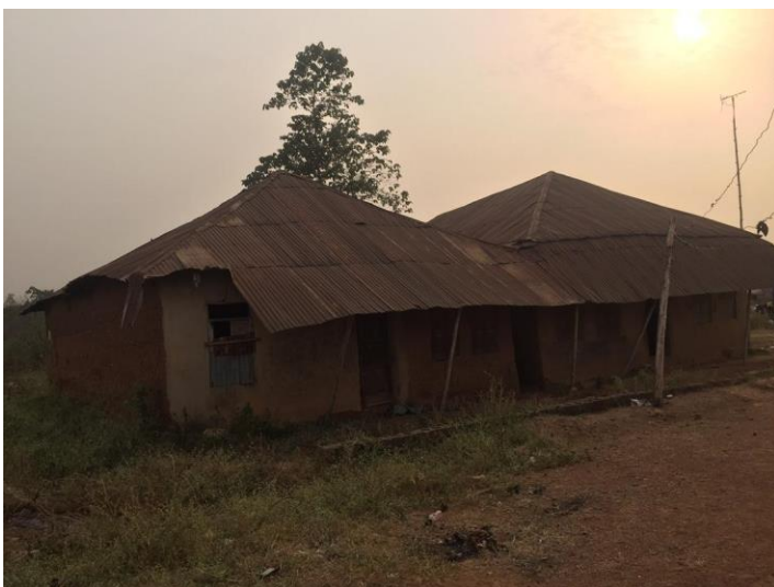
Fig 2- photograph showing building under study on the right with the “uninhabited twin” on the left.
